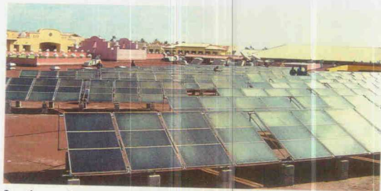
Over the past five years, Transsen has built more than 250 large-scale systems in Brazil, Chile, Peru, Argentina and Bolivia. The majority of those systems were used in hotels and multi-family homes.
